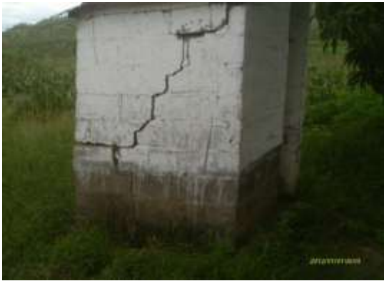
FIGURE 2: Cracks on the latrines walls and floors
