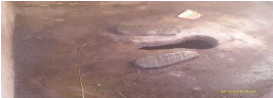
FIGURE 9: Dirty latrine with blood stains
