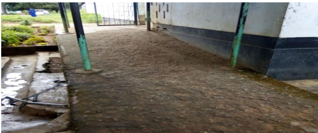
Figure 15: A dormitory ramp at Dudu/Teka (Source: Field data, 2018)
