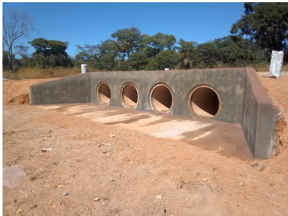
Figure 6: Structure along the terminated project road not protected from erosion
