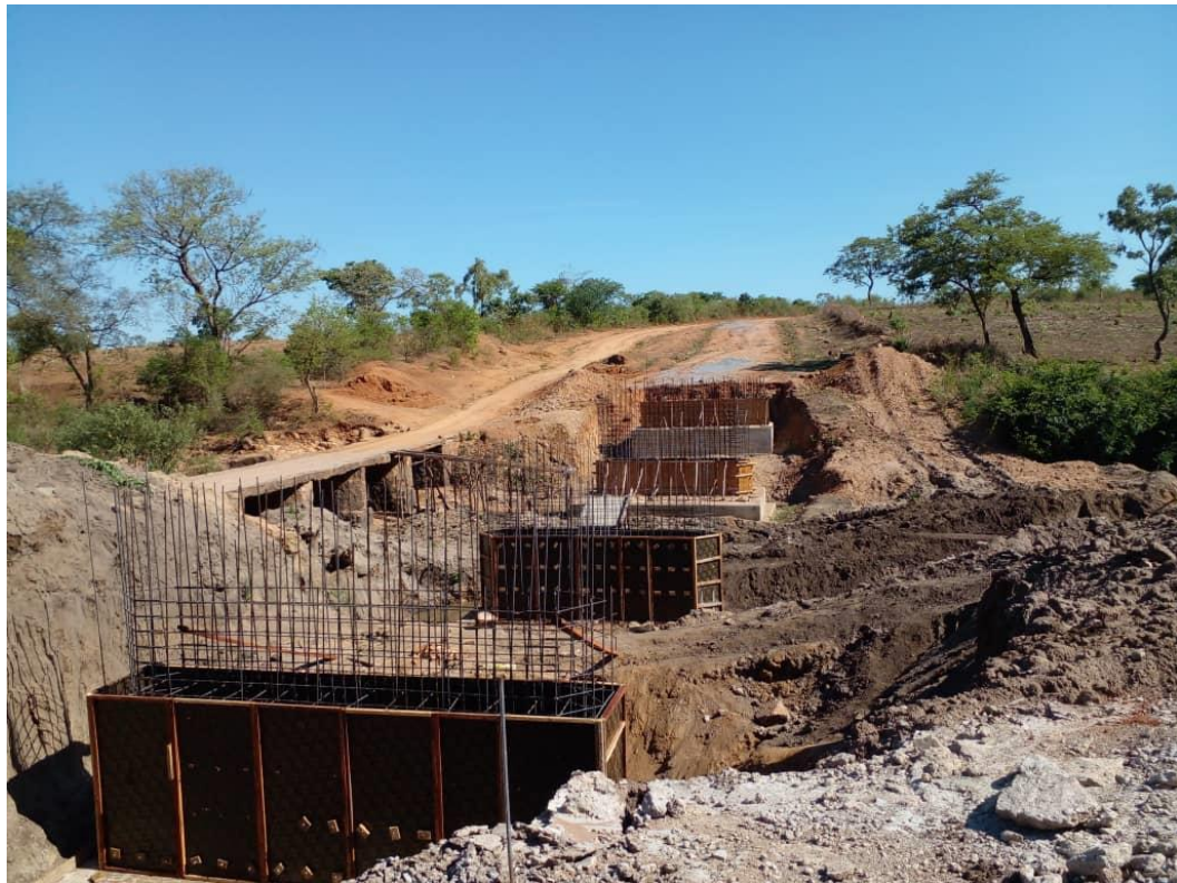
Figure 7: State of Msanzala Bridge after contract termination
