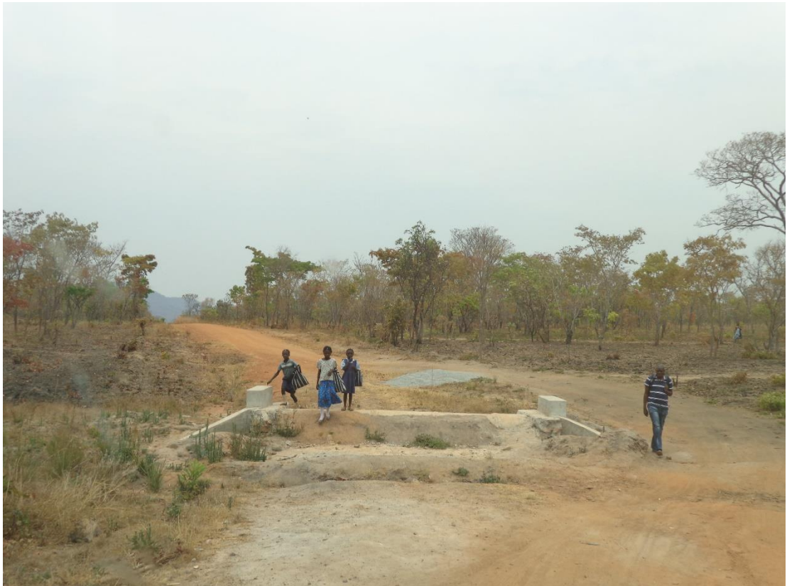
Figure 8: A section of the abandoned road showing an exposed installed pipe culvert
