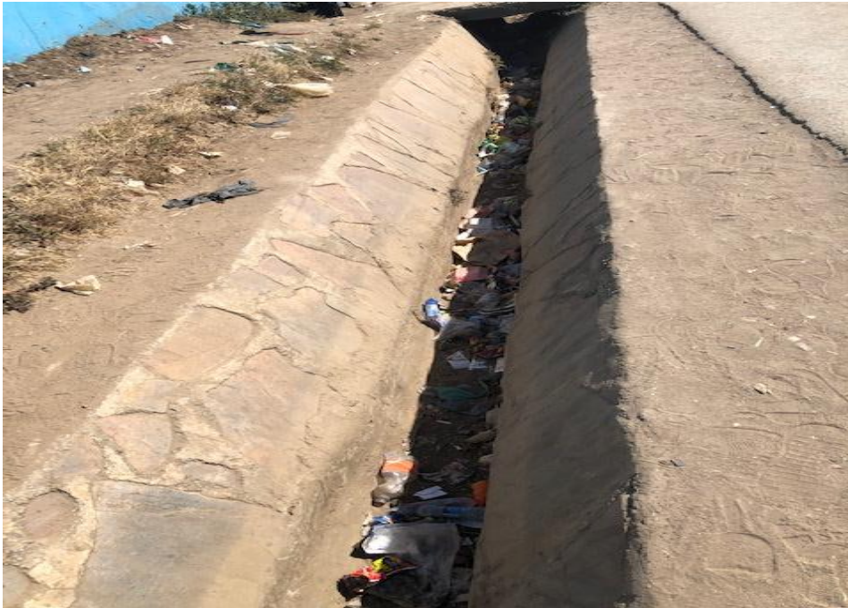
Figure 11: Indiscriminate disposal of waste in the drainage Source: Field data 2021.
