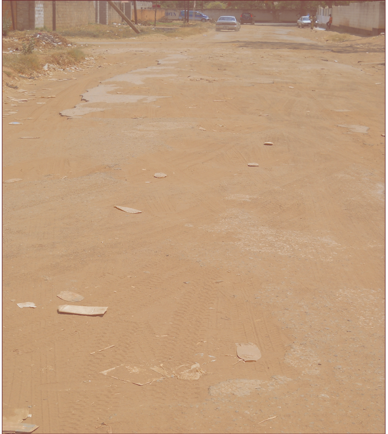
PHOTO 7: Deteriorating road in Kabwata Ward (forming junction with Burma Road at Lutheran Church)
