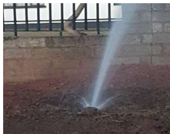
Figure 4.2: High system pressures
