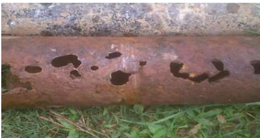
Figure 2.15: Corroded underground steel pipe (Source: LWSC NRW Strategy, 2014)
