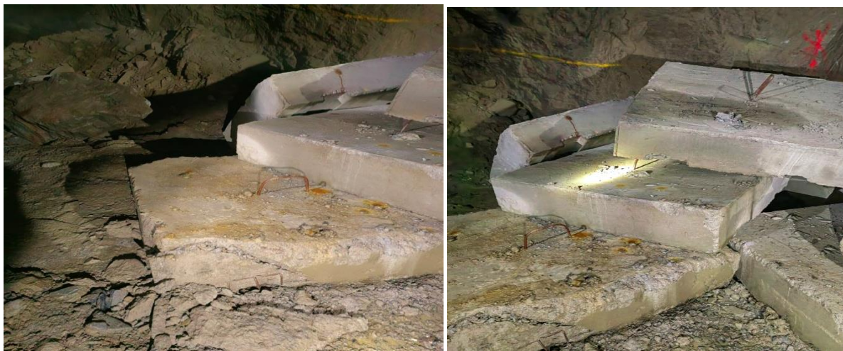
Figure 3.15: Crushing of the poorly constructed concrete packs
