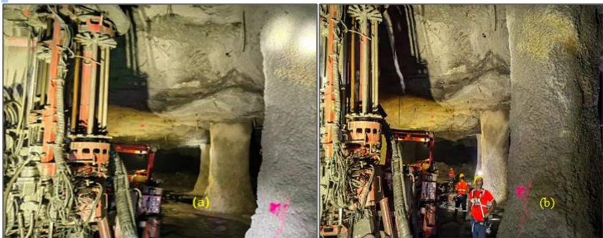
Figure 3.13: Condition of the artificial concrete pillars during longhole drilling
