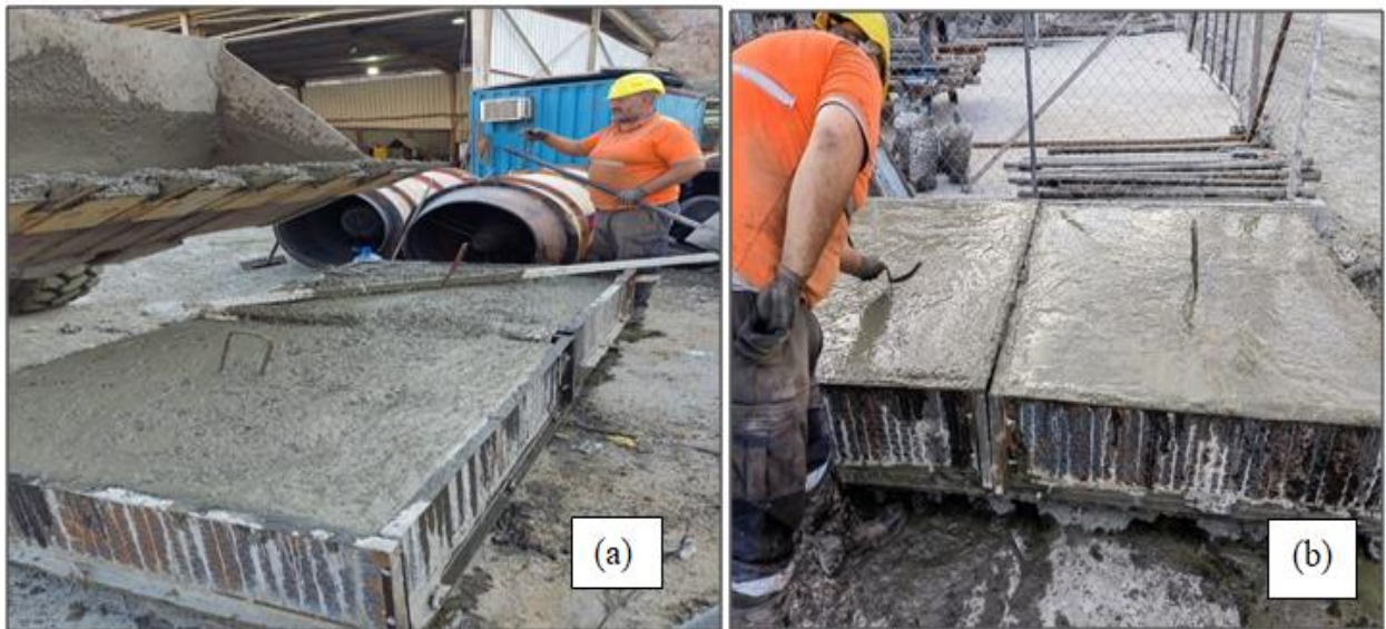
Figure 3.10: Pouring of the mixed concrete into the mold (a) and operator distributing the concrete (b)
