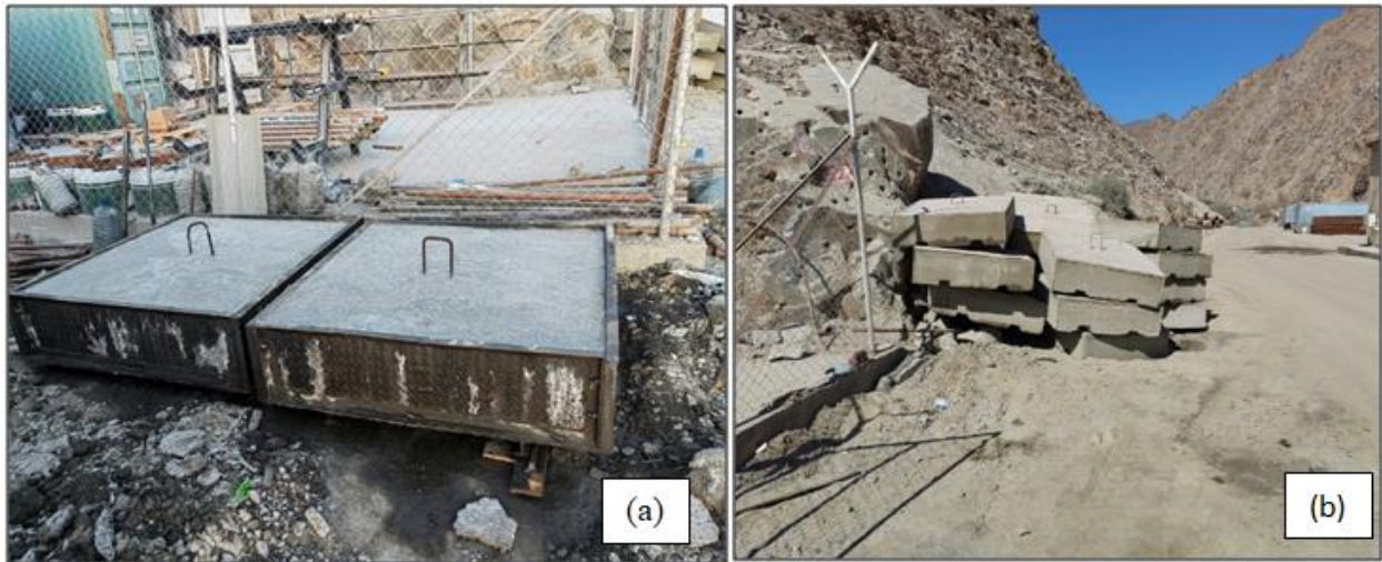
Figure 3.11: Concrete pack constructed before being removed (a) and constructed concrete pack ready to underground.
