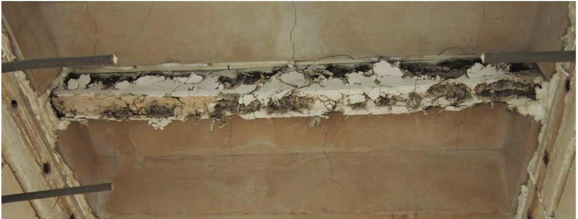
Figure 3.2: RLF2-20 beam inside the furnace after the fire test. Extracted from (Kahanji, 2016)
