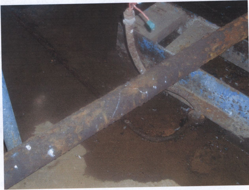
Fig 9: Corroded Pipes at UNZA-GER campus
