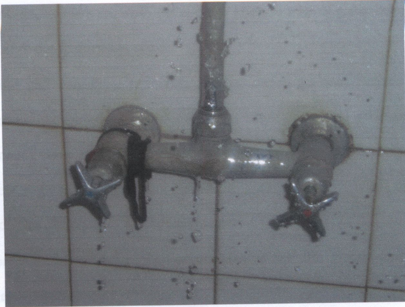
Fig 10: Water leakages from a shower mixer at UNZA-GER
