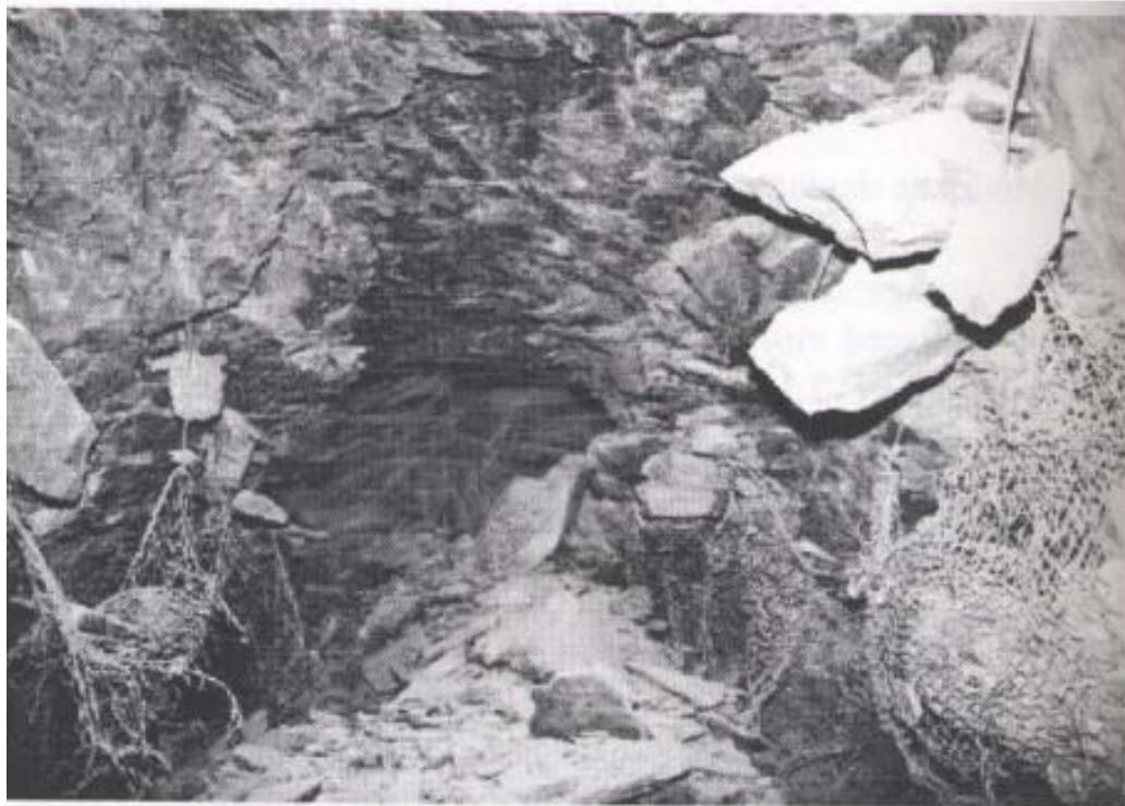
Figure 2.5: Major Rockburst damage resulting in closure of the drift (Kaiser et al., 1996)
