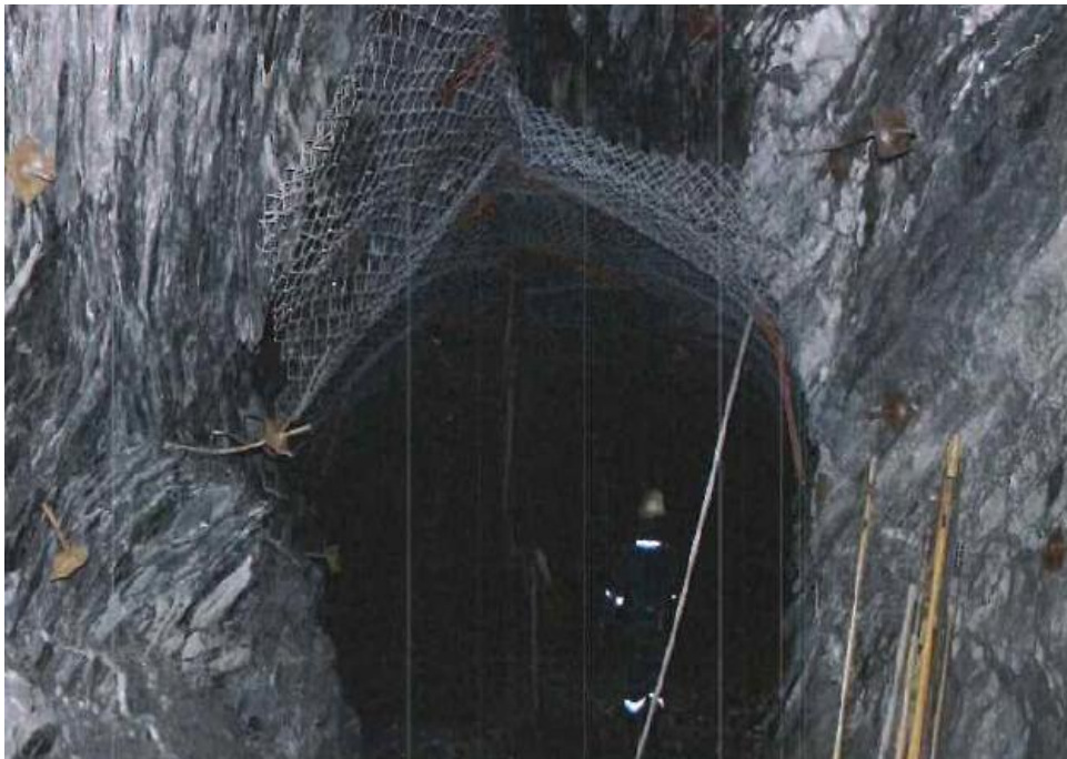
Poor ground conditions on 3510 level - buckled sidewalls under stress
