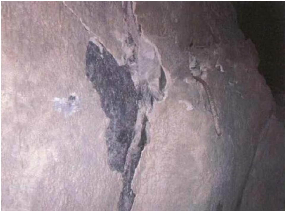
Poor shotcrete support- Thin and cracked (3360 HLGE)
