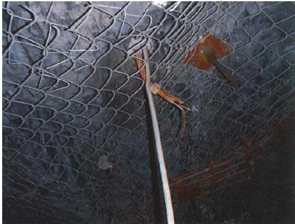
Poor Cable Bolt Support on 3510 level - No face plate
