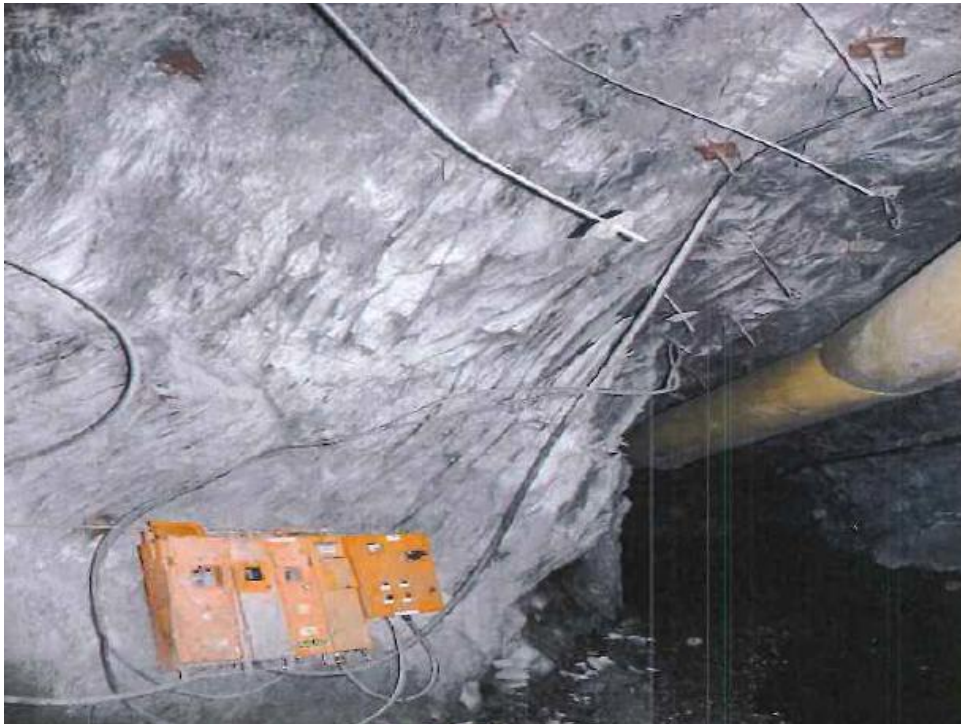
Poor Cable Bolt Support on 3360 level - protruding Bolts
