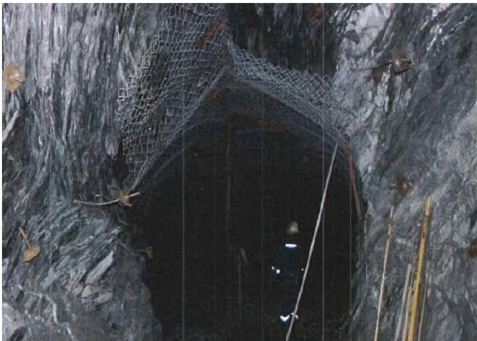
Figure 1.2: Highly stressed and sheared ground on 3860 Level
