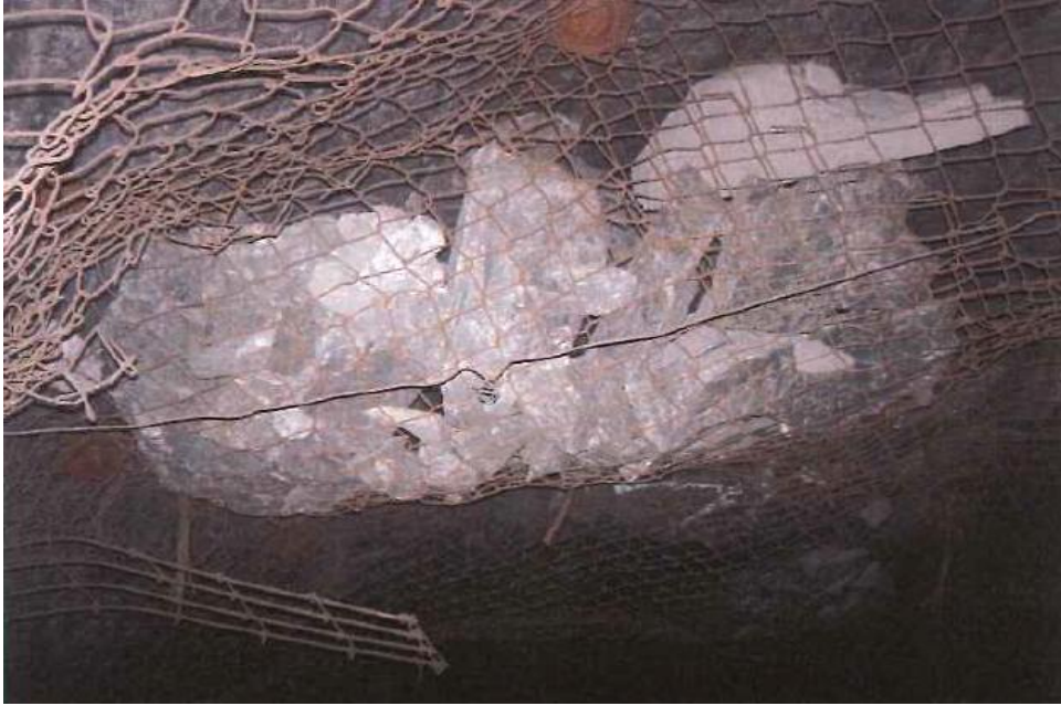
Poor Mesh Support on 3510 level
