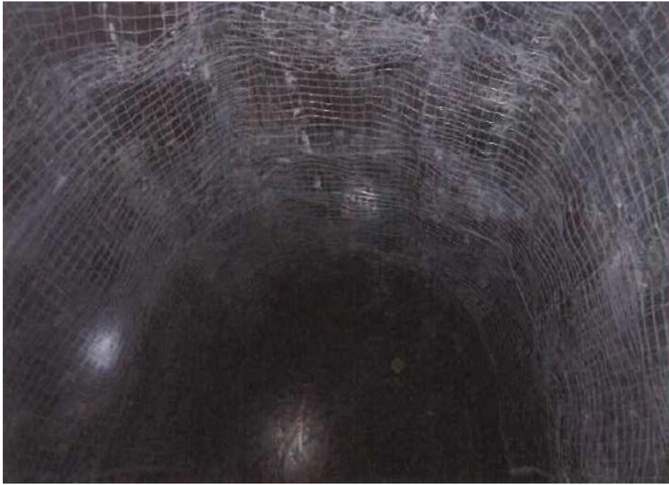
Good Mesh Support on 3760 level - Tight against rock walls
