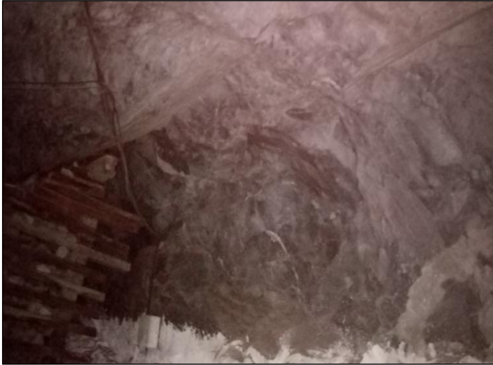
Poor Timber support on Central Shaft 3360 Level (Tilted and One-sided)
