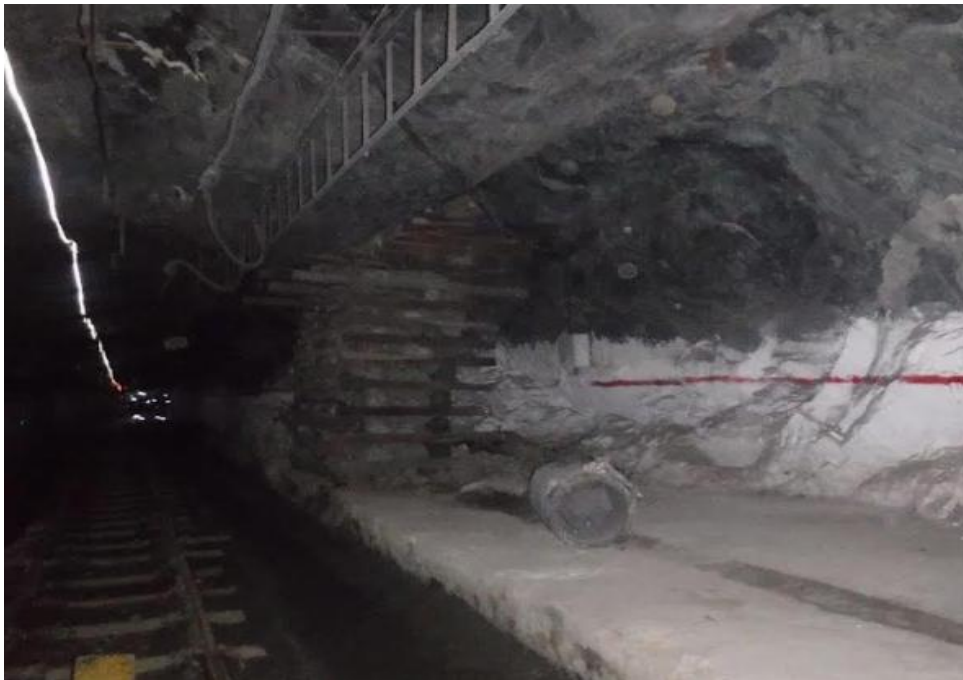
Poor Timber support on Synclinorium/SOB Shaft 3360 Level (One-sided)
