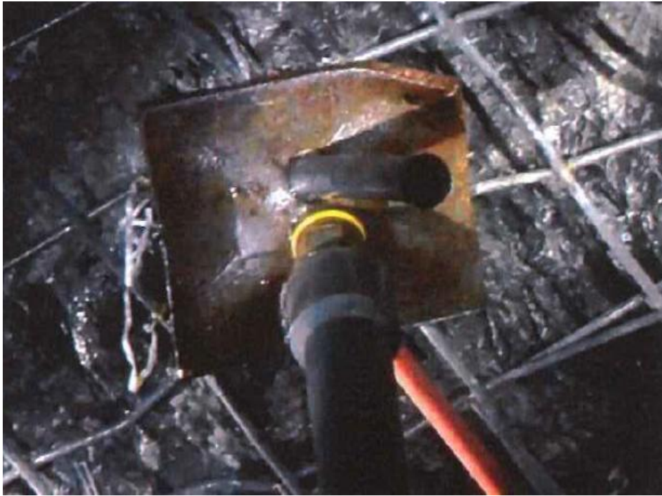
Good Cable Bolt Support on 3510 level - Load indicator showing yellow
