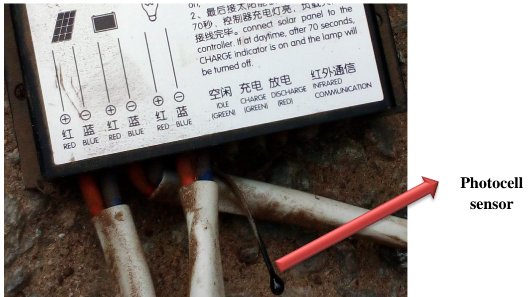
Figure 15: Solar charge controller with an embedded photocell sensor
