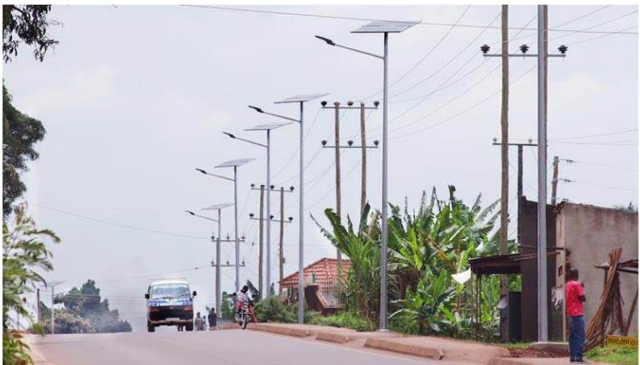
Figure 5: Solar-powered street lights in Kampala, Uganda. [49]
