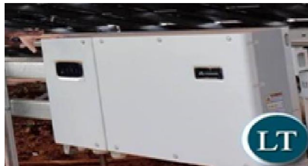
Figure 4.12 Huawei - 480-volt Inverter from Bangweulu Solar Power Station
