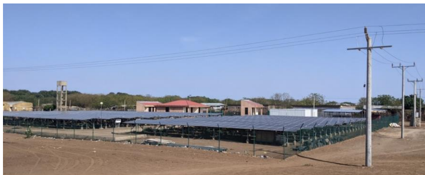
Figure 4.4 A view of the PV MG infrastructure in Omorate, Dasanech district, Southern Ethiopia
