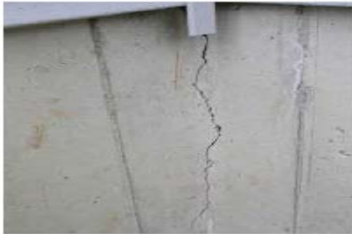
Figure 32: Cracks forming in some houses of Wusakile
