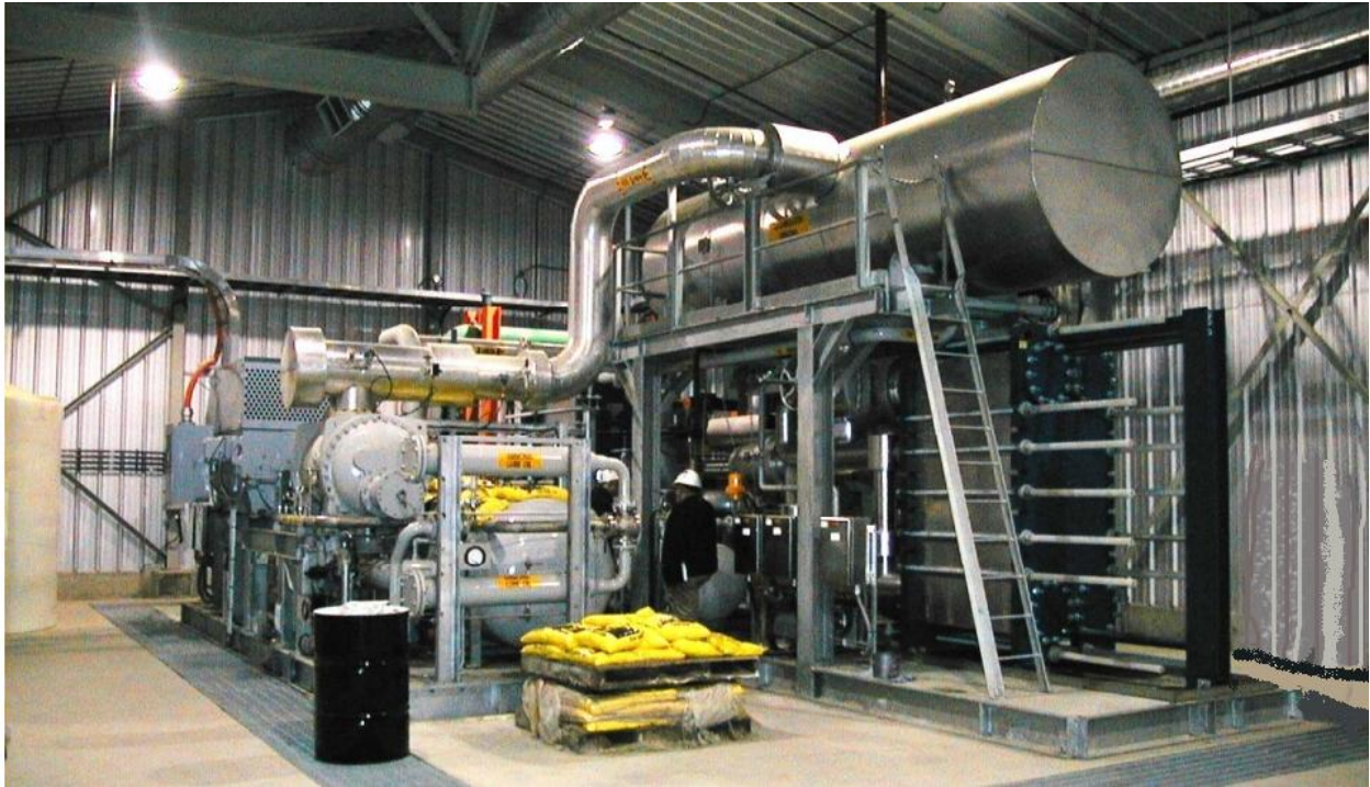
Figure 40: Surface refrigeration supplying cold water underground (Ramsden & Von Glehn, 2012)
