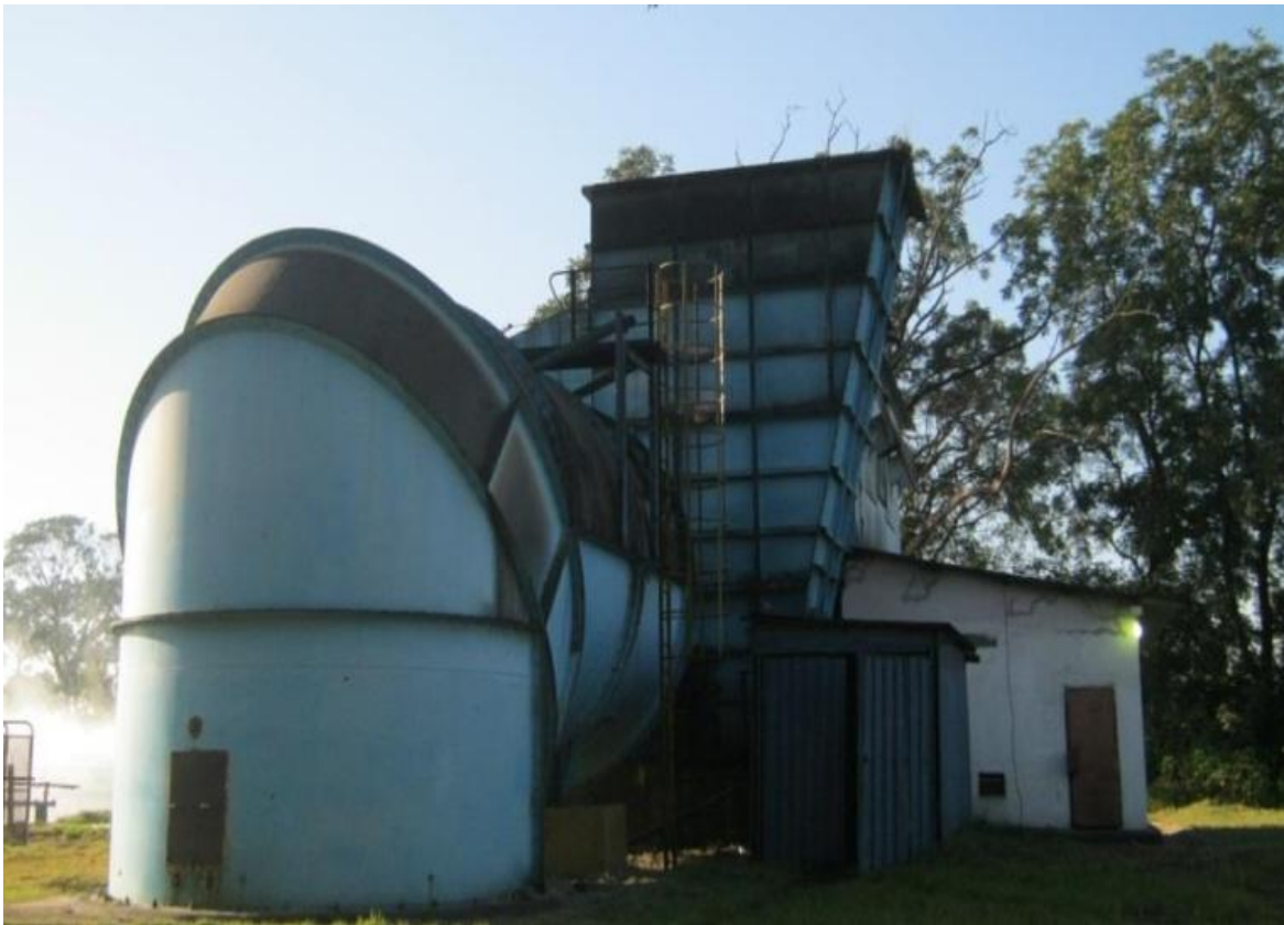
Figure 21: V10 Main Upcast Fan
