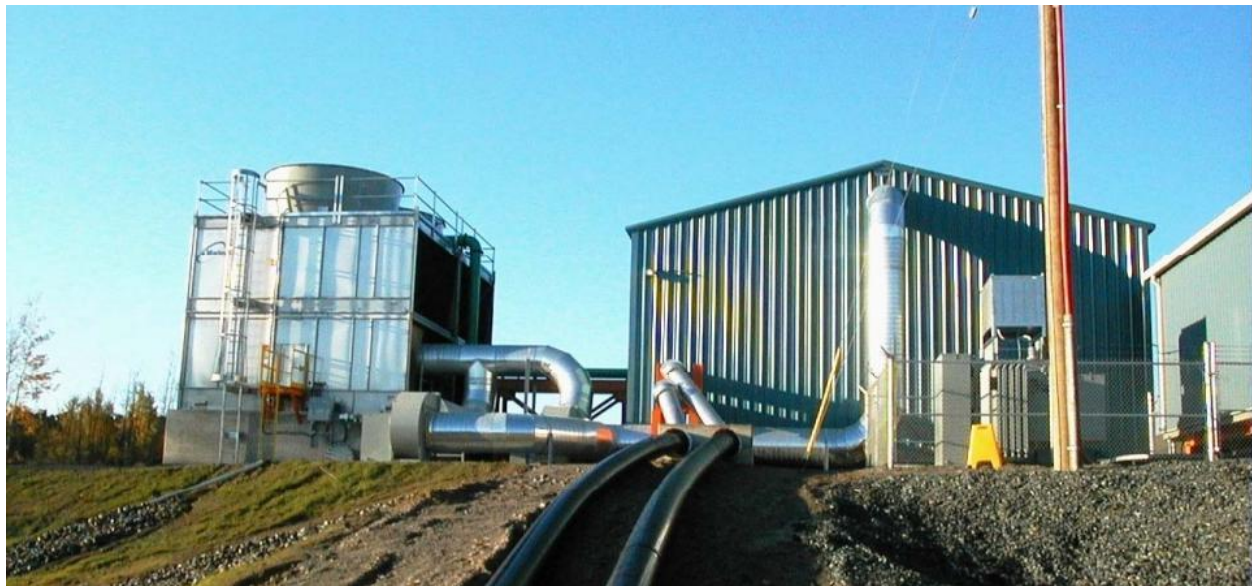
Figure 39: Surface refrigeration plant (Ramsden & Von Glehn, 2012)
