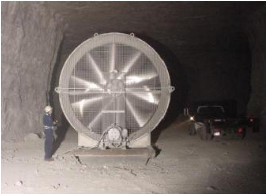
Figure 8: Booster fan used to transport and dilute dust (Chekan, 2010)
