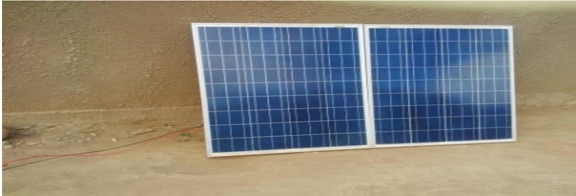
Figure 5.4 (c): Solar panels used during load shedding
