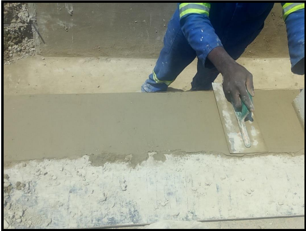
Figure 4.14: Picture showing exposure to wet concrete on the road project
