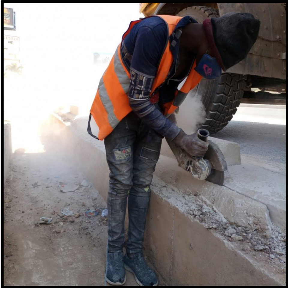
Figure 4.34: Picture showing a worker without adequate PPE
