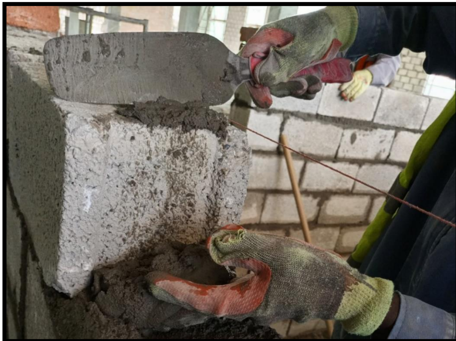
Figure 4.17: Picture presenting exposure to wet mortarduring building
