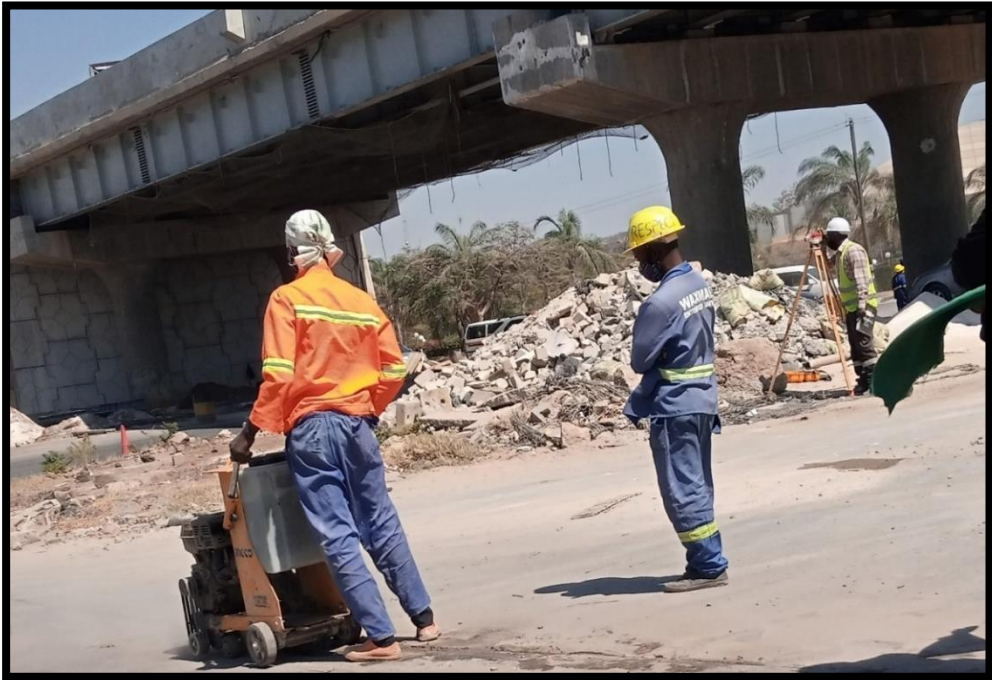
Figure 4.25: Picture showing the use of cutter with water on the road project
