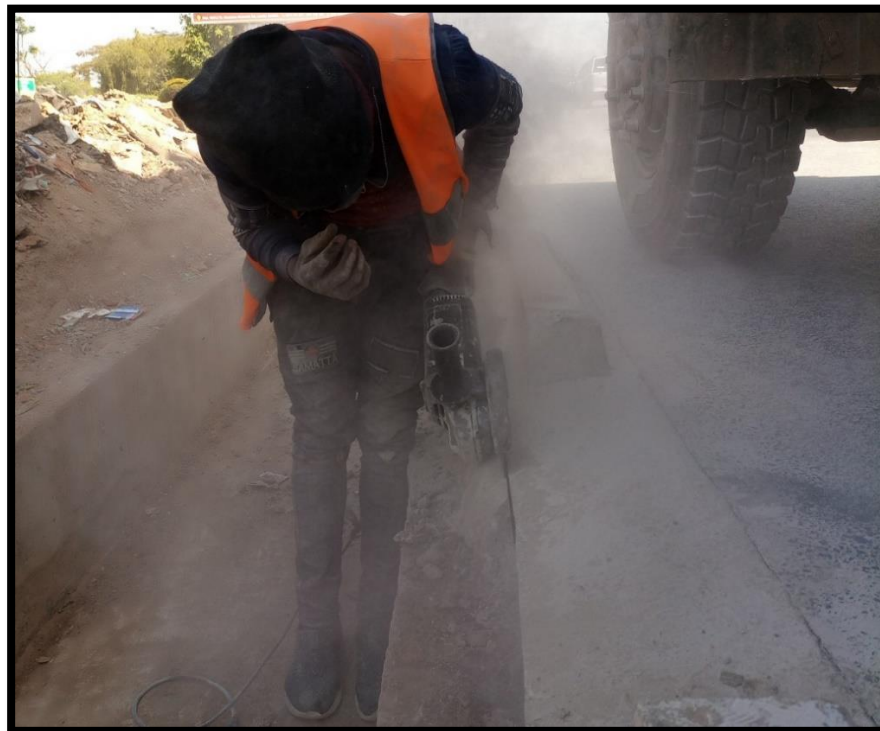
Figure 4.9: Picture showing dust exposure during dry concrete grinding
