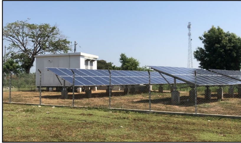
Figure 2-3: Yoma Micro Power solar-hybrid power plant in rural Myanmar [Source: Norfund]
