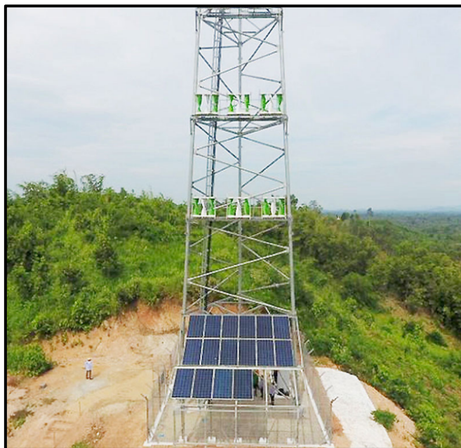
Figure 5-1: Telecommunication towers built in off-grid areas (source: edotcogroup.com)
