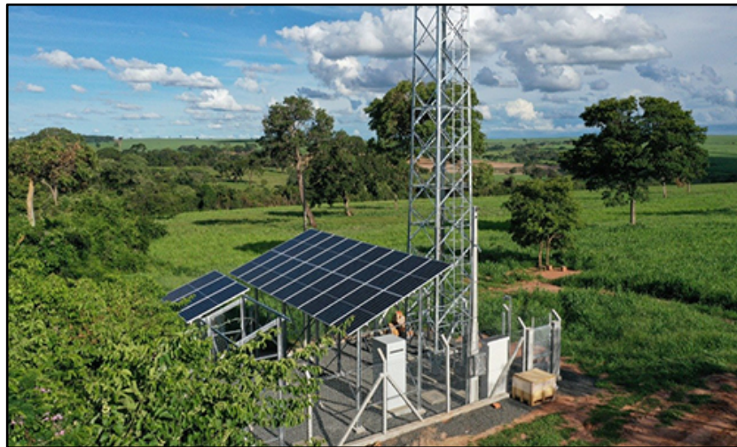
Figure 2-2: iSAT off-grid Solar System
