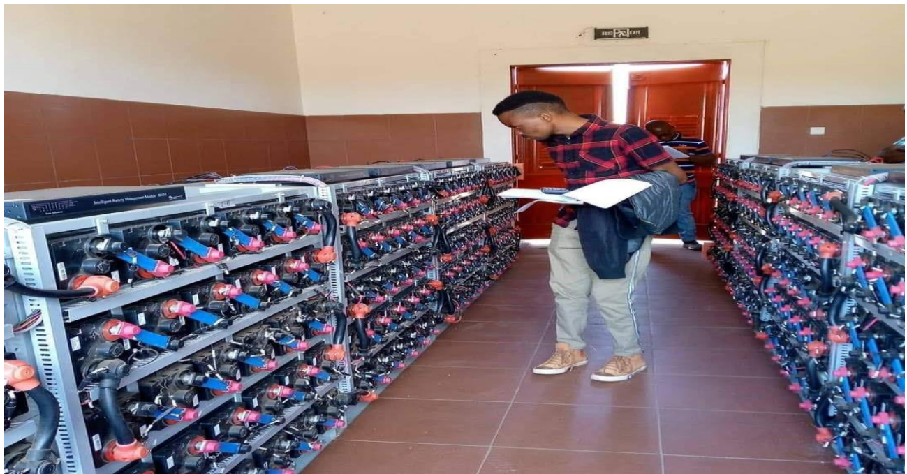
Figure 1: Katamanda Solar Mini-Grid Battery bank
