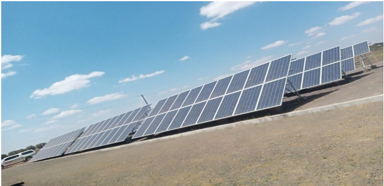
Figure 11 Katamanda solar mini-grid PV configuration
