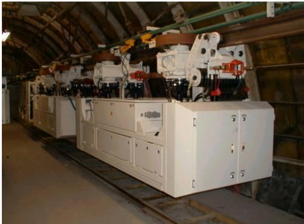
Figure 2.6: Monorail train power pack (Scharf, 2007)
