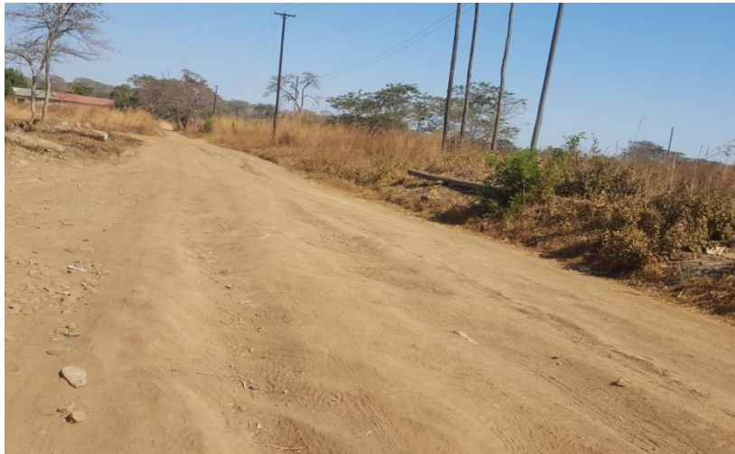
Plate 2: Condition of a road in Mpongwe
