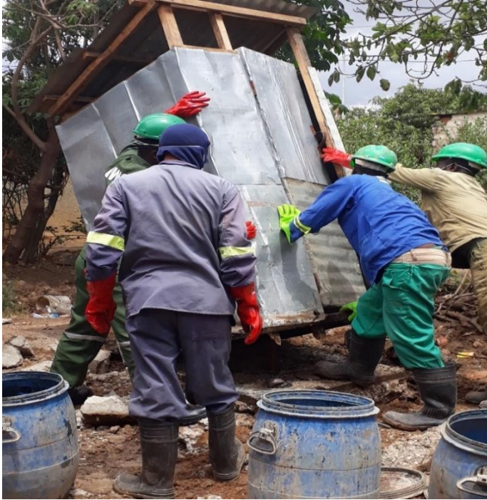
Figure 19: Latrine being demolished during emptying, an example of poor design (Source: Author, 2018)
