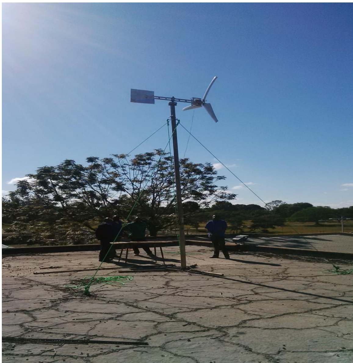
Figure A2.3: The Hybrid being mounted at the School of Engineering.
