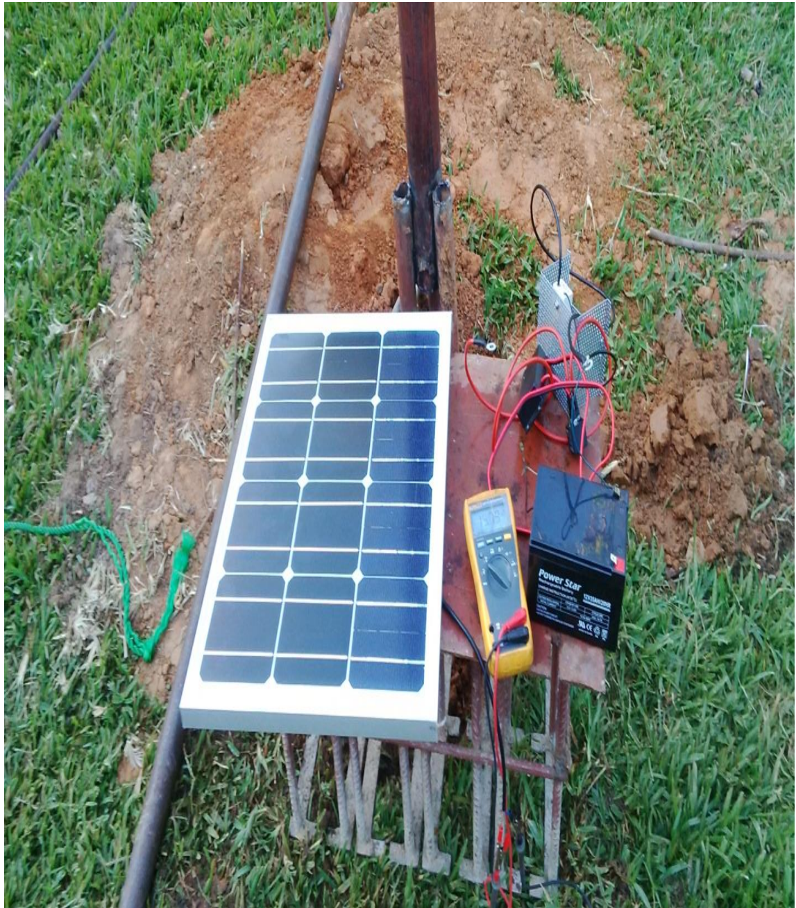
Figure A2.2: The Solar Panel, Converters and the Battery.
