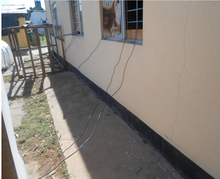
Figure 4.4: Pictorial view of cables extending to the dryer.
