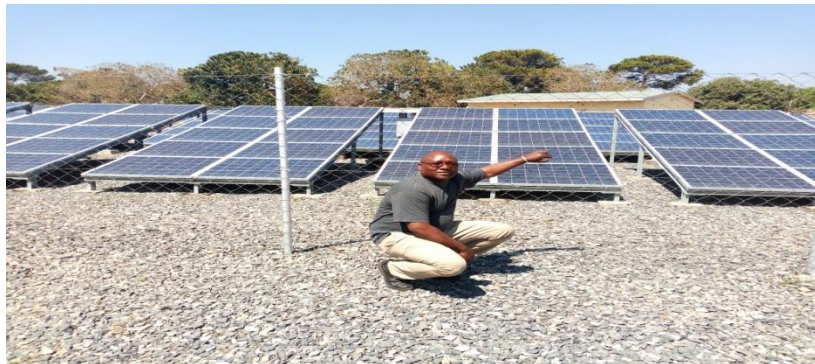
Figure 4. 24: Picture of solar modules array at Mpanta SMG
