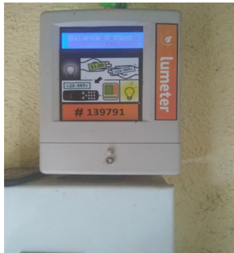
Figure 4. 7: Picture of installed prepaid meter in Sinda village
