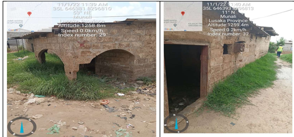
Figure 18: House in Mtendere Township sinking with passage of time: House has sunk by 0.8m within past 4 years (Courtesy: Owner Mr. Mwanza)
