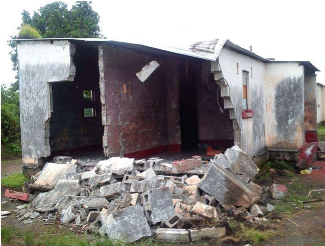
Figure 2: Picture showing one of the collapsed houses in Chingola (Source: Zambia National Broadcasting Corporation (ZNBC) News Online 23 rd November, 2021)
