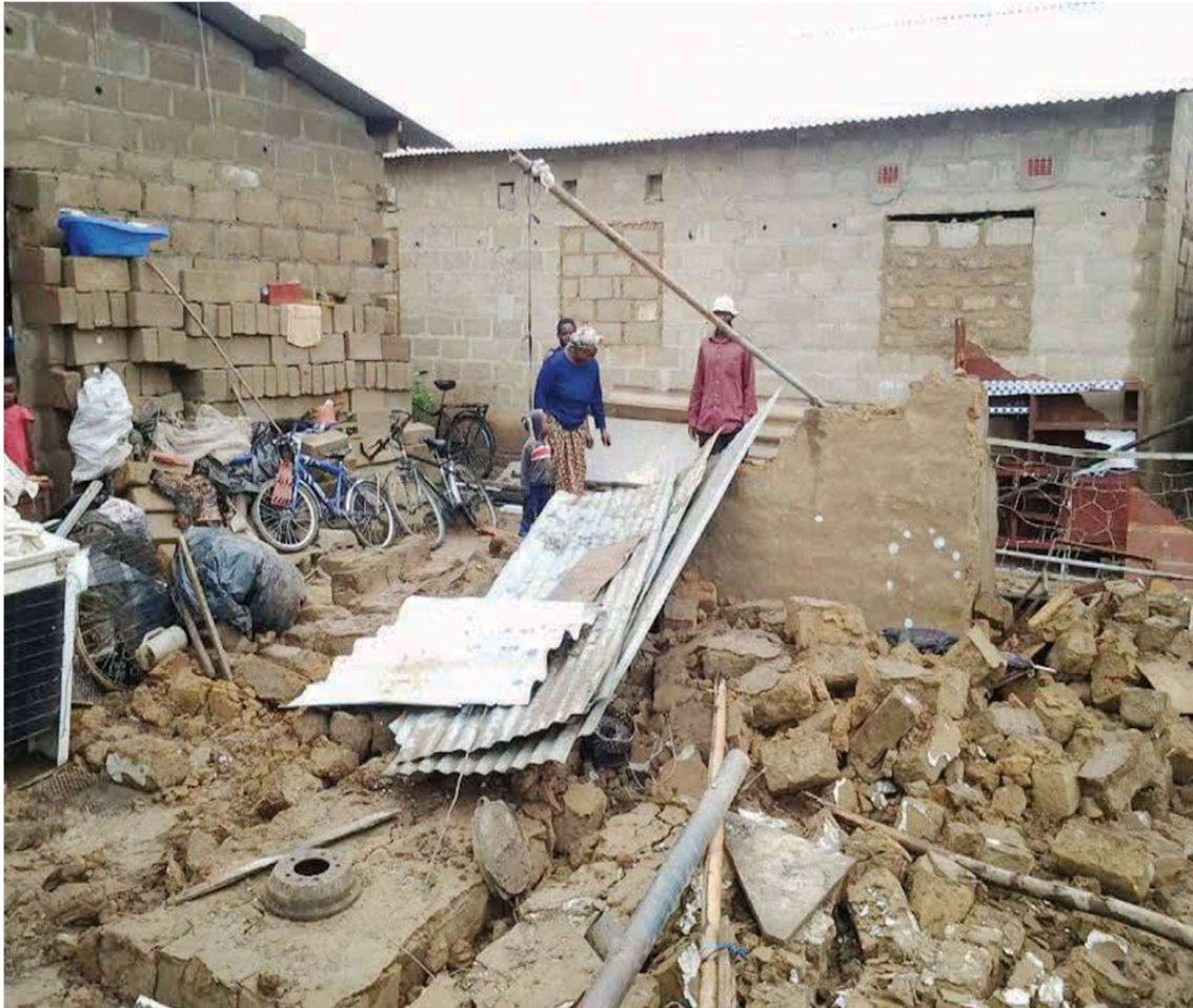
Figure 1: Collapsed house in Mazabuka (Source: Zambia Daily Mail News 24 th December, 2014)
