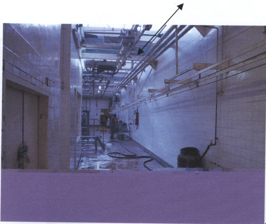
Figure 6. 4: Overhead conveyor rails
