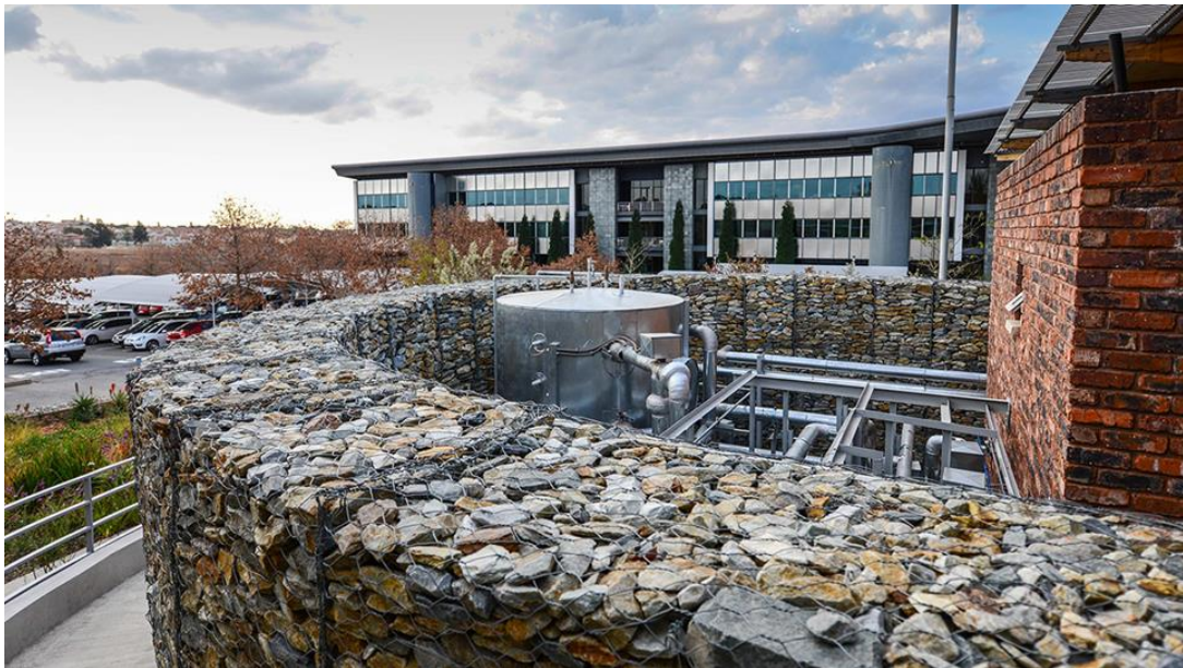
Figure 4.1-6 Solar Absorption Chiller
