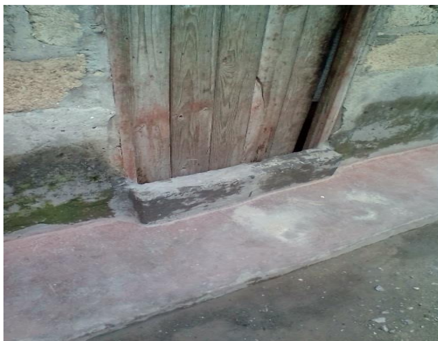
Figure 9: Raised doorstep used to prevent flooding water
