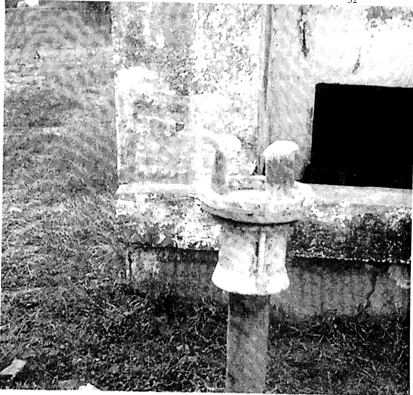
Figure 3.3 shows a broken under drain nozzle
