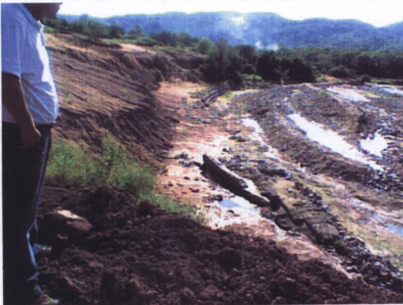
Figure 5.4: Damage to embankment of Lusaka – Chirundu road
