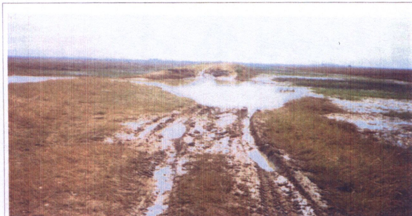
The Mongu –Kalabo Road is almost non existent
