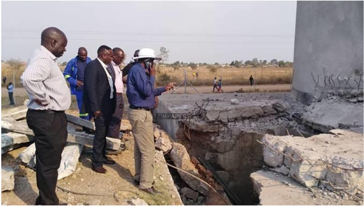
Figure 2.1 Damaged depot in Zimbabwe (Source: Herald Newspaper)
