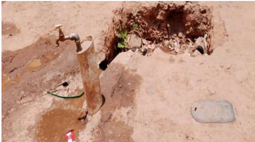
Figure 11: Vandalism of the pipe which takes water to the tap.
