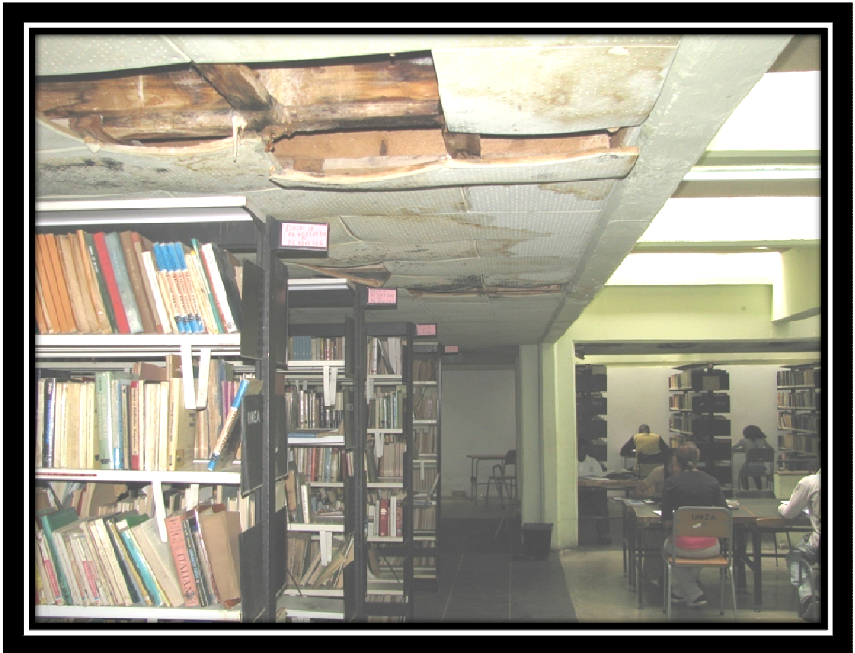
Figure 5: Falling ceiling board due to rain water leakages in the Main Library
