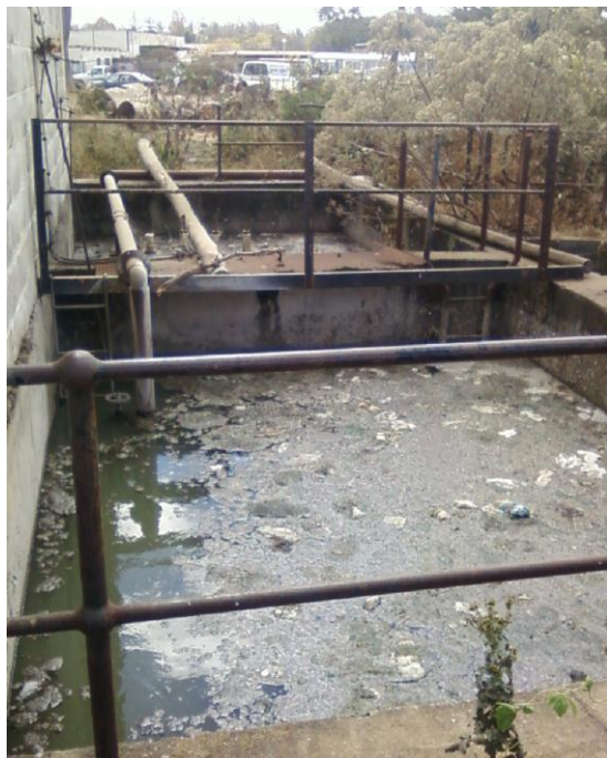
Figure 5.12: UNZA sewerage main processing plant near Transport Yard.
