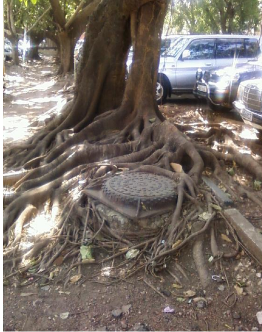
Figure 5.7: Manhole under a rubber tree in Car Park B by School of Natural Sciences.
