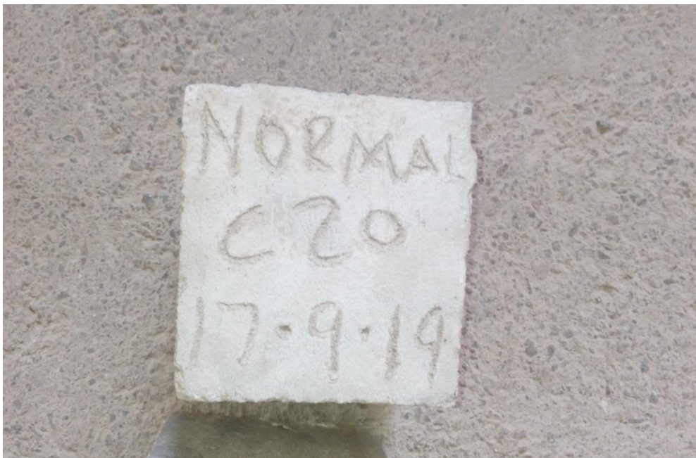
Figure E.2: Normal concrete not exhibiting cracks after being subjected to heat at 100 ° C for 48 hours
