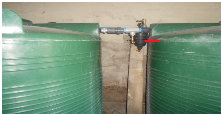
Figure 18: Showing a filter between storage tanks in Luumbo area, Gwembe District, Southern Province, Zambia
