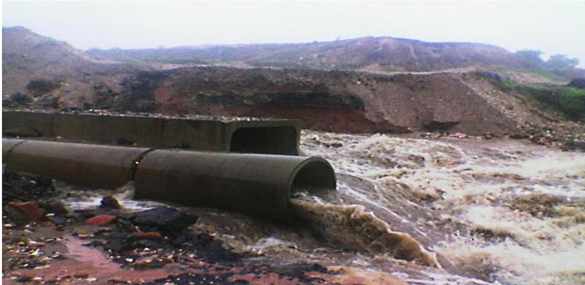
Figure 4.2 Washed-away Izuma “B” Bridge due to heavy rain, 2007
