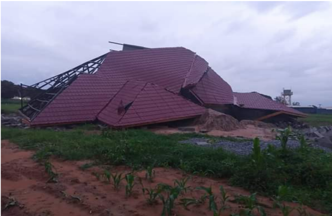
Figure 7. Image shows one of the demolished houses by the Lusaka province minister.
